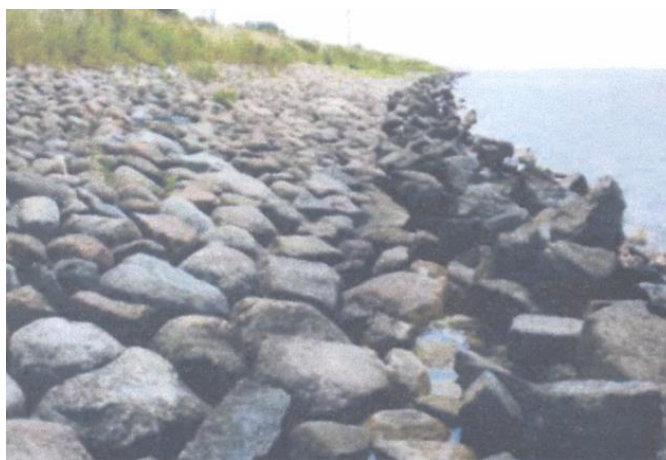
Figure 4.1.4 Armour layer consisting of pitched stones (left) and randomly dumped stones at toe (right)
